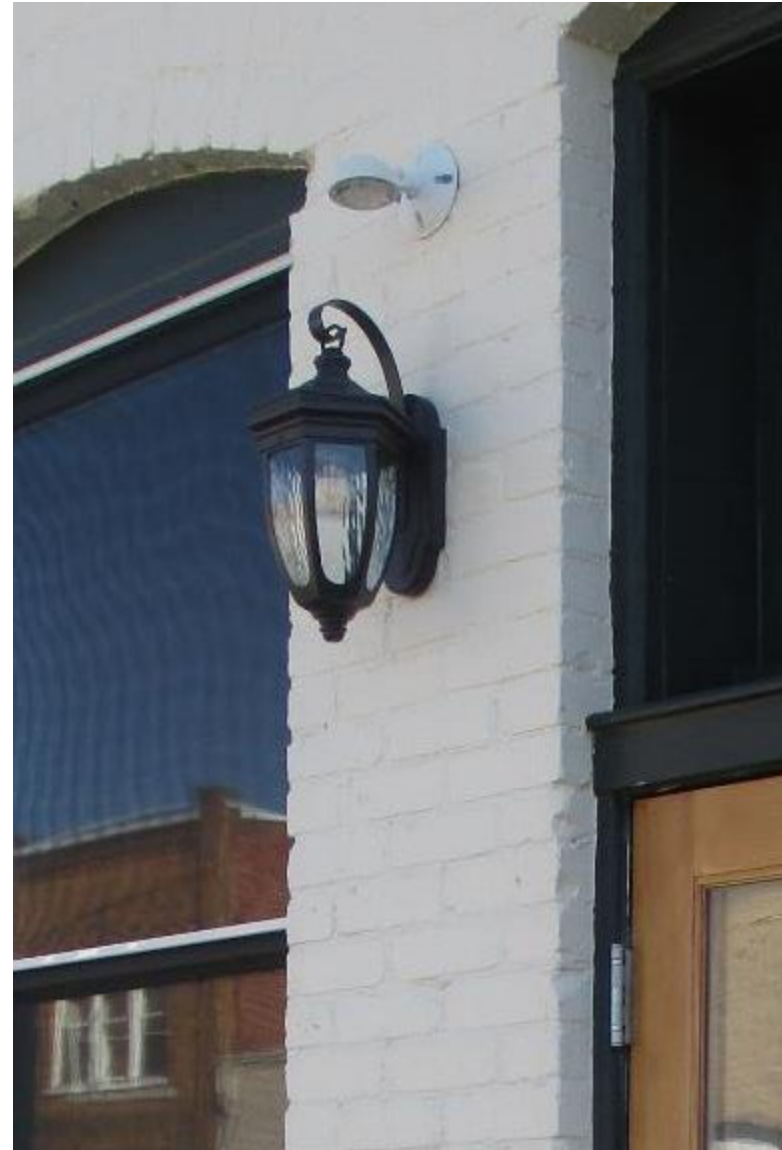
Photograph 51: Contemporary exterior lighting should be compatible with the historic architectural features of the building.
