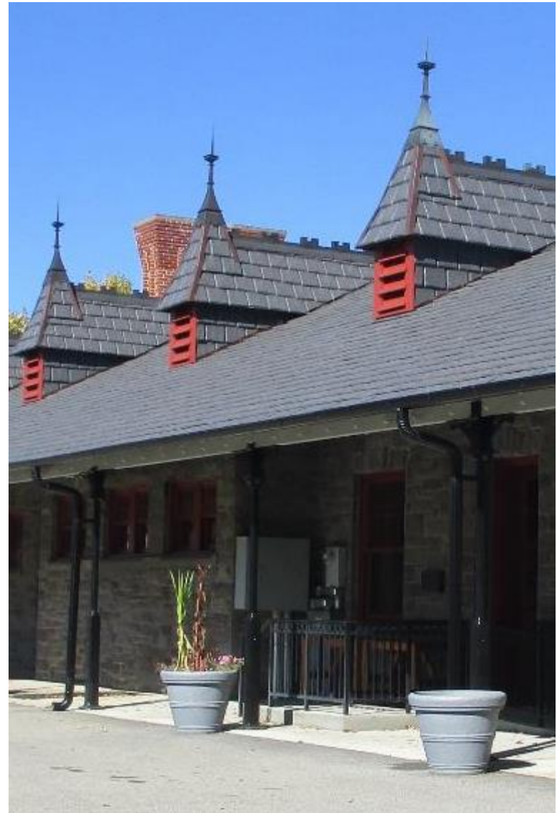
Photograph 24: Many historic buildings have gutter and downspout systems that are integrated with the building's design.
